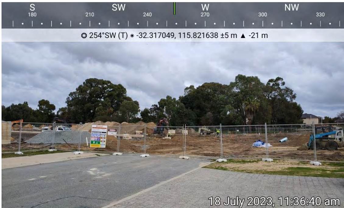
Plate 2: Evidence of construction internal road network and connection to external road network is underway and internal site being cleared.
