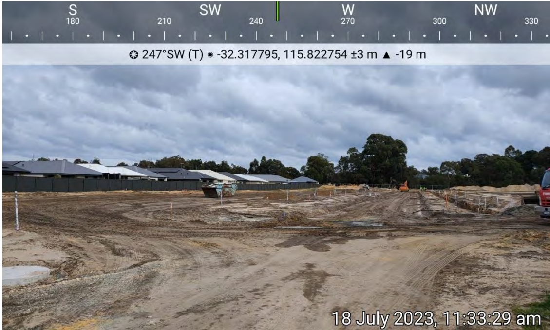
Plate 1: Evidence of construction internal road network is underway and internal site being cleared.
