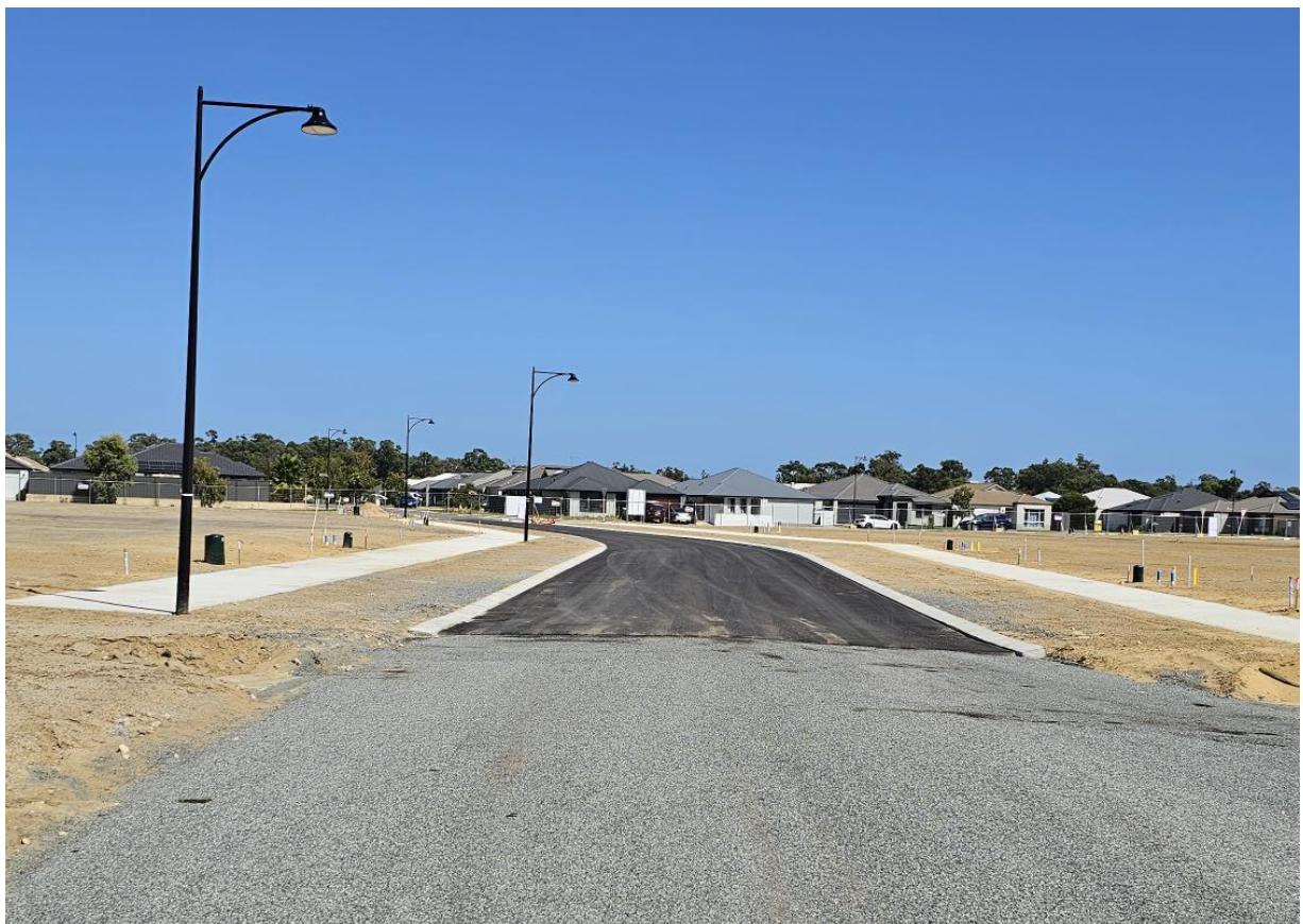
Plate 6: Evidence of construction of roads and temporary cul-de-sac turn around area in accordance with Roadworks layout plan (Frasers Property Australia Photo).
