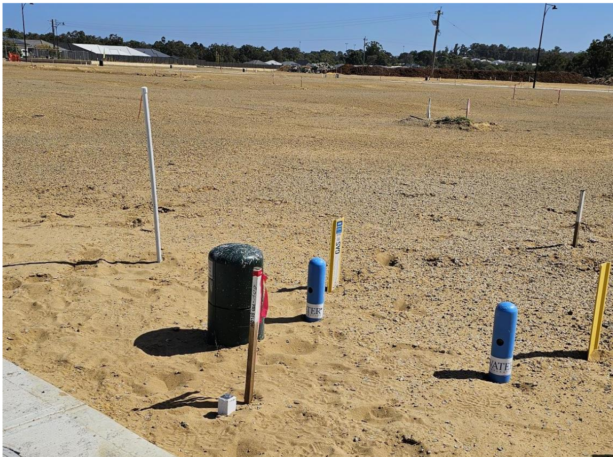
Plate 8: Evidence of installation of reticulated water within construction site is underway. (Frasers Property Australia Photo).
