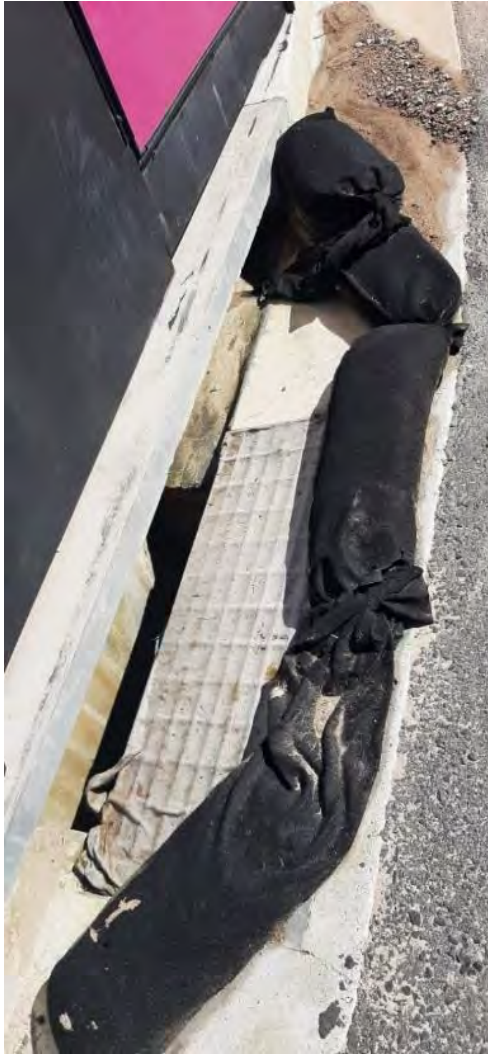
11. Silt bags and fabric filter installed around stormwater drain downstream from work site.
