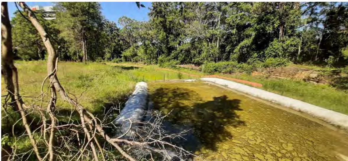
16. Secondary sedimentation basin with overrun into third basin and eventually grass.
