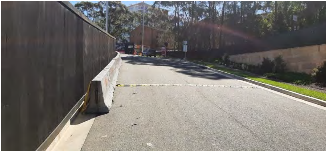
17. Clean access way with A class hoarding installed around construction works preventing dust and debris escaping the work zone. .
