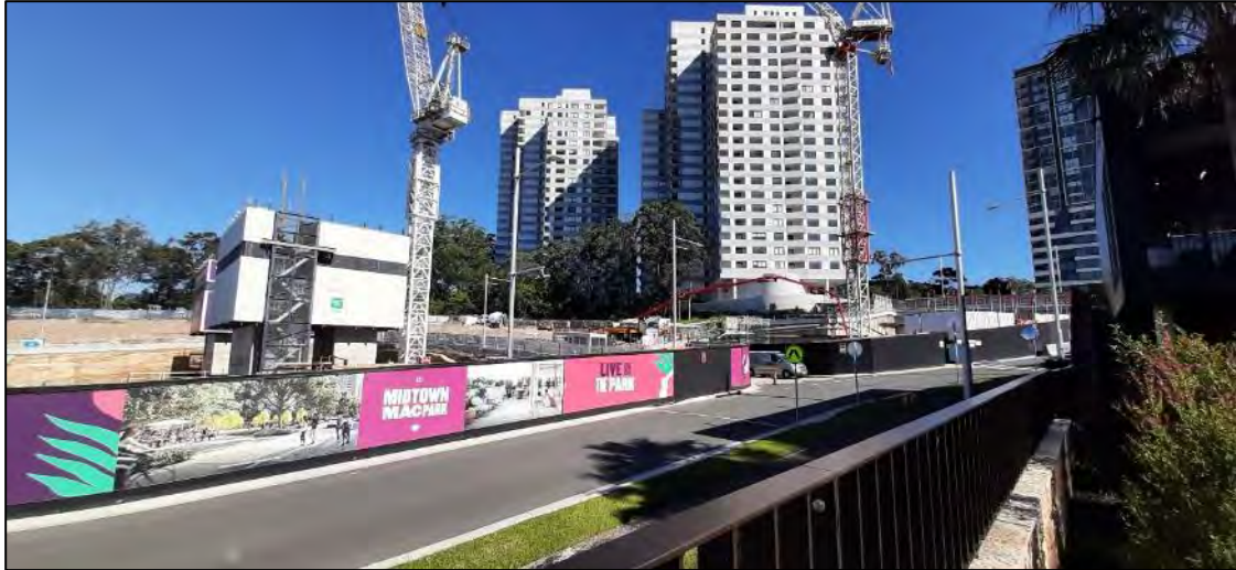
1. Facing west from sales and display centre carpark towards basement construction works for the A1 building (right) and C1 building (left).
