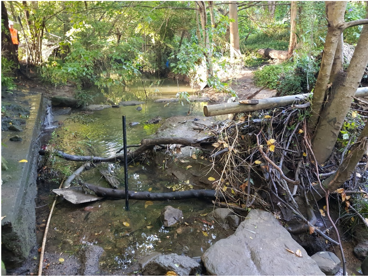
Figure 2: Debris and Obstructions in Creek Channel
