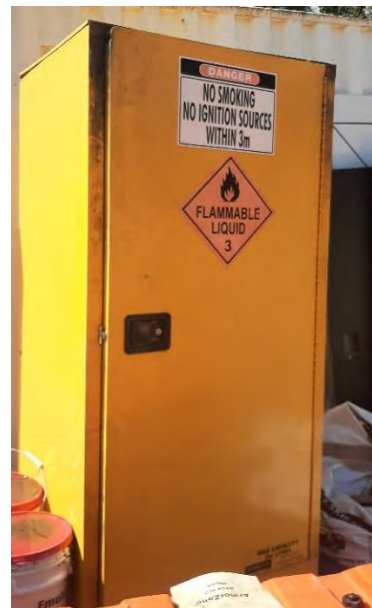
22. Unlocked storage for flammable liquid.
