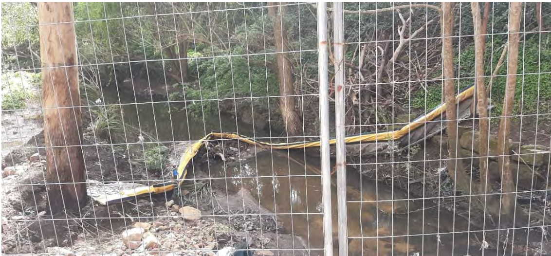
17. Shrimpton Creek – downstream. Buoyant sediment trap full of debris.
