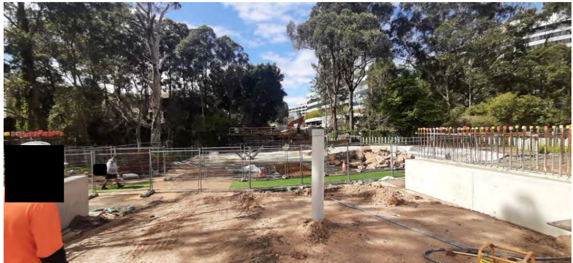
14. Construction over Shrimptons Creek crossing, piling and reinforced concrete slab – facing southeast.
