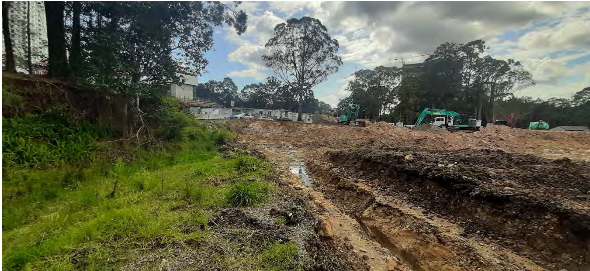
7. Excavated swale for temporary diversion of upslope stormwater along the southwestern boundary of the site – facing northwest.
