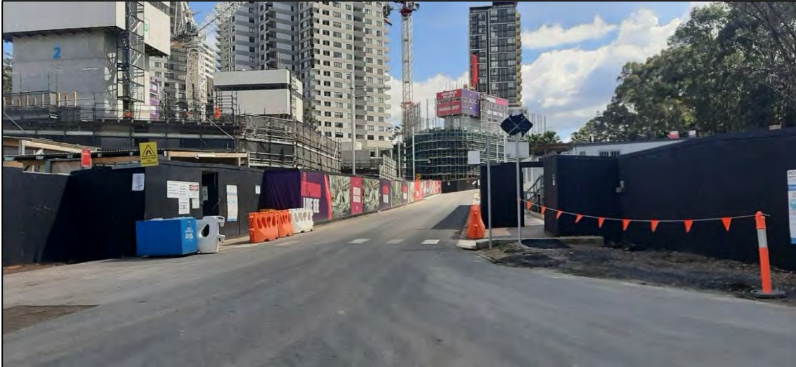
27. Access Road (Road No. 1) from Stage 1B work site to Herring Road – facing northwest towards Herring Road.
