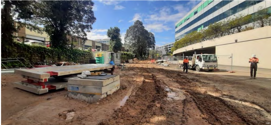
19. Temporary laydown area for inert bridge construction material south of Shrimptons Creek – facing southwest towards Lyonpark Road.
