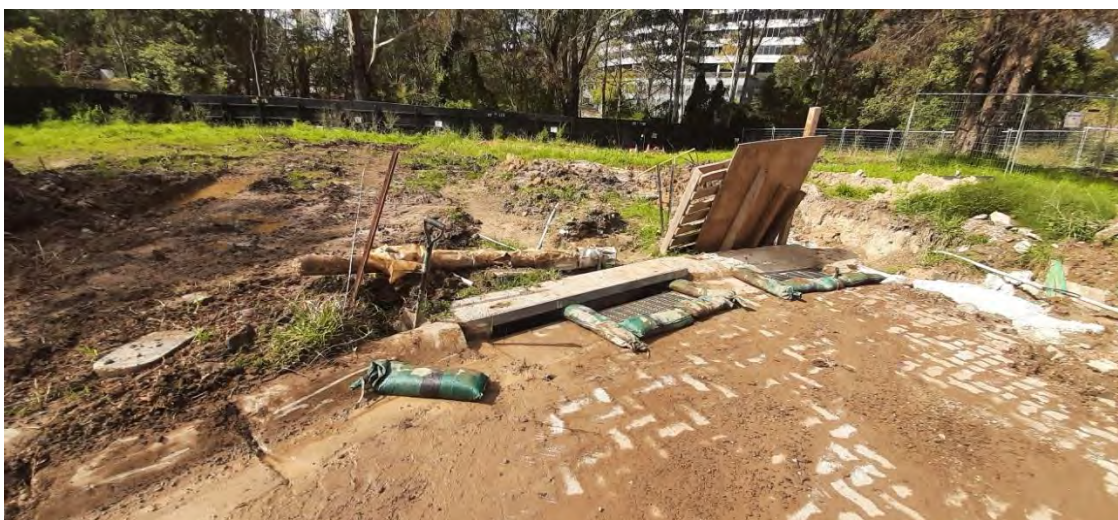
15. Signs of uncontrolled sedimentation around stormwater drain in the south south the site adjacent to Shrimpton Creek.
