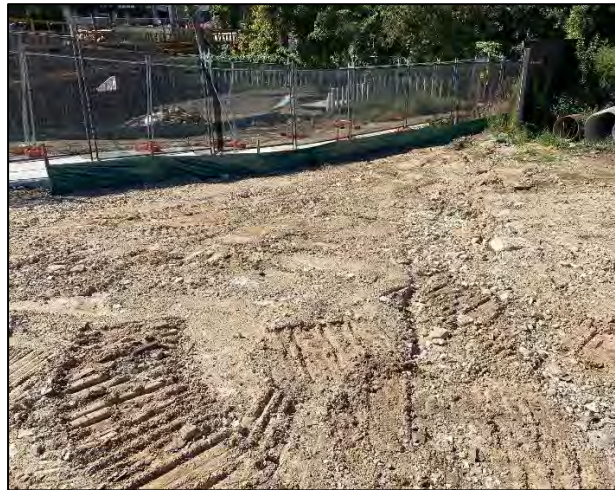
14. Additional silt fence and shade cloth installed along footpath to the south of the site 31/03/2023.
