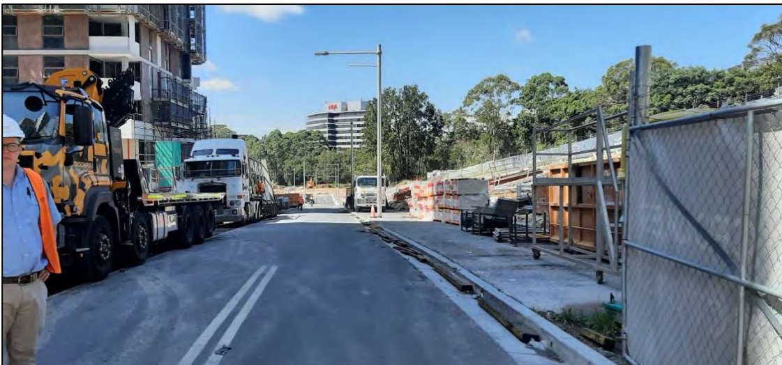
5. Road No. 2 facing southeast - Richard Crookes construction to the left in the photograph. 15/03/2023
