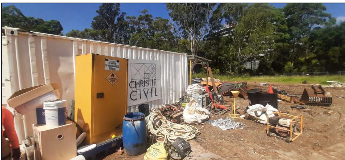
19. Hazardous storage area to the south of the site. 15/03/2023
