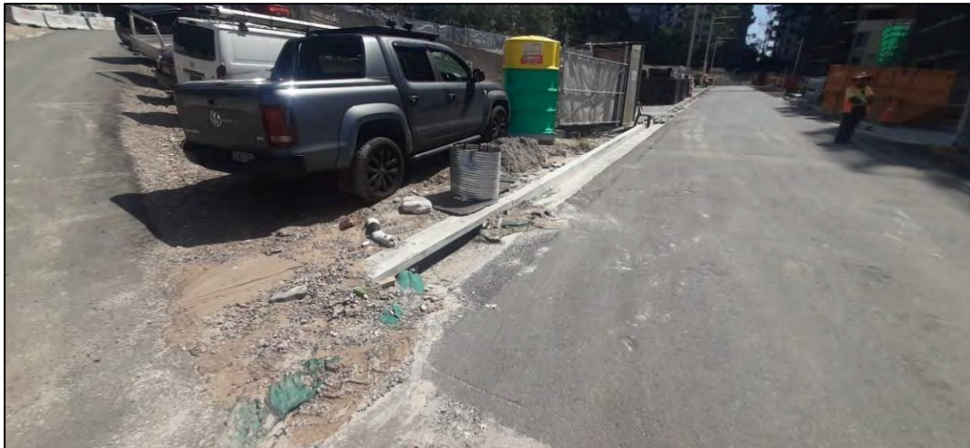
7. Signs of uncontrolled erosion and sedimentation around stormwater drain along Road 2 to the south of Richard Crookes Construction site below parked vehicles. 15/03/2023
