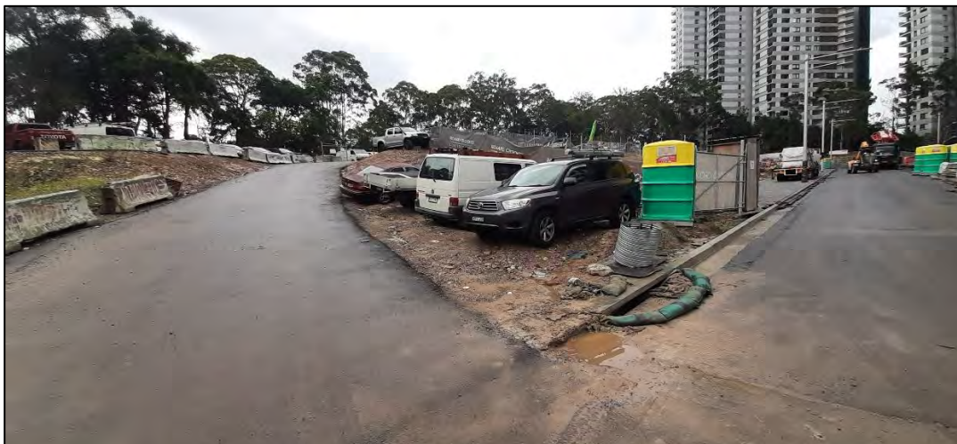
8. Silt bags reappplied around stormwater drain along Road 2 to the south of Richard Crookes Construction site. 29/03/2023
