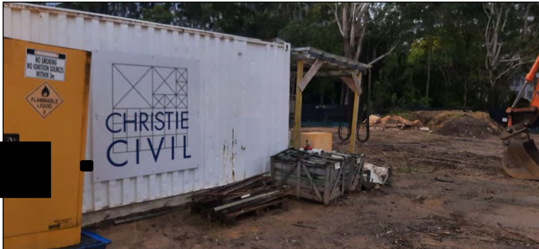
20. Hazardous storage area to the south of the site tidied up. 29/03/2023
