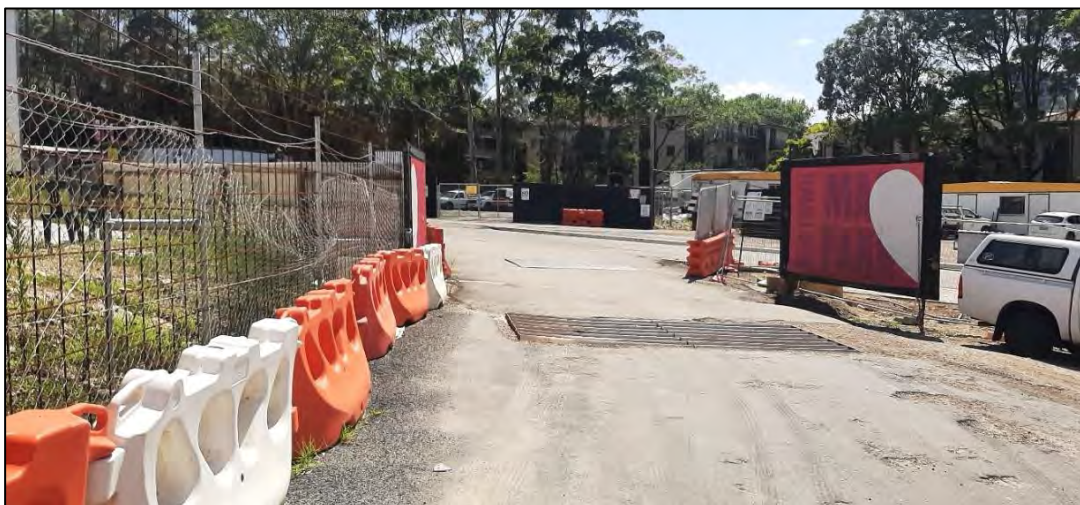
9. Heavy vehicle entrance / exit to work site – facing north towards Road 1. Shaker grid in foreground and Christie site office beyond. 15/03/2023
