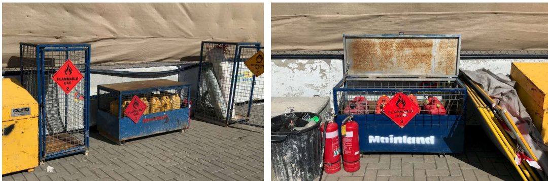
Figure 4.7.6.1.2– Spare Fuel Contained in Bunded Flammable Cages
