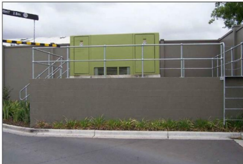
Figure 51 - Example substation raised above 1:100 flood level
